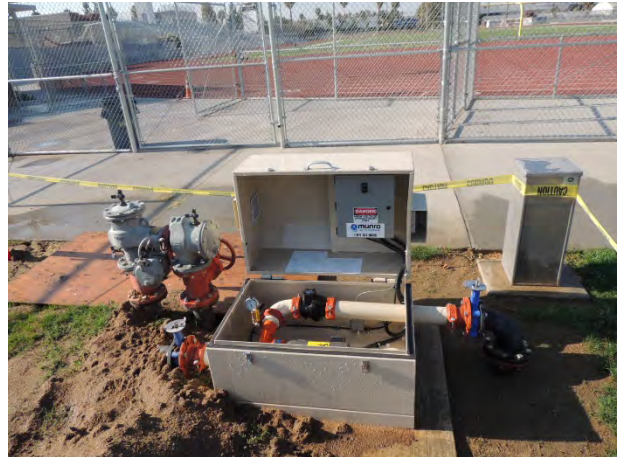
Field Cooling Booster Pump
