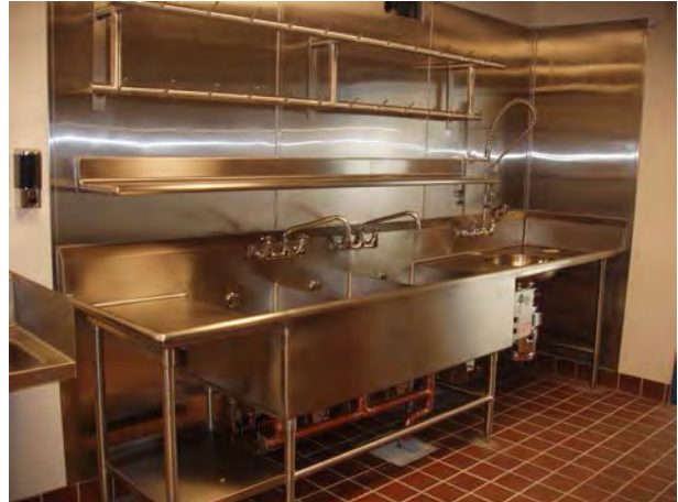
New Kitchen Sinks
