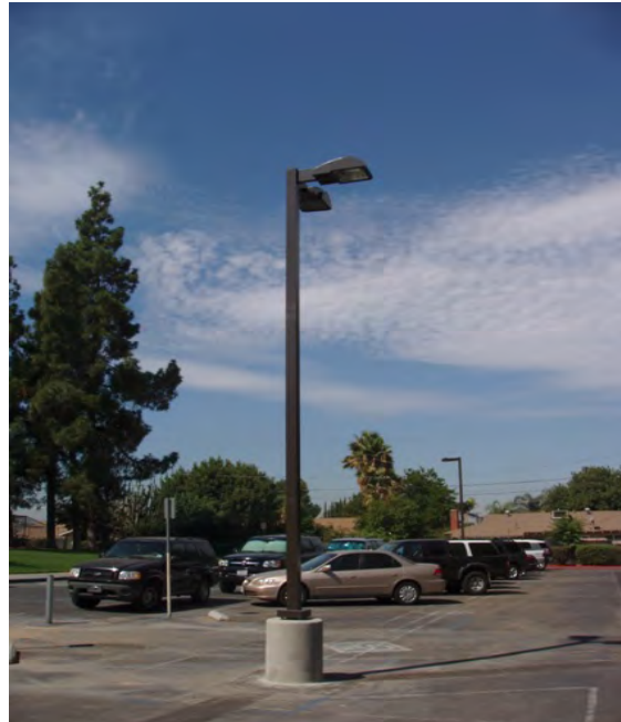
New Parking Lot Lighting
