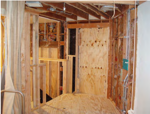
MPR top of stage wheelchair lift platform
