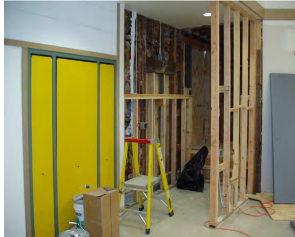
MPR front view of new wheelchair lift entry point
