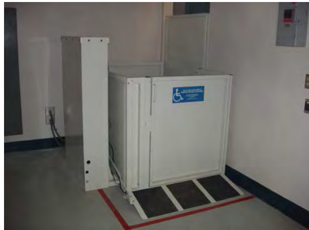
New Wheelchair Lift in the MPR
