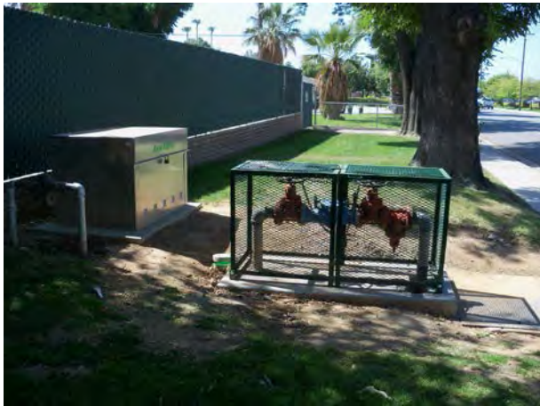
New Booster Pump
