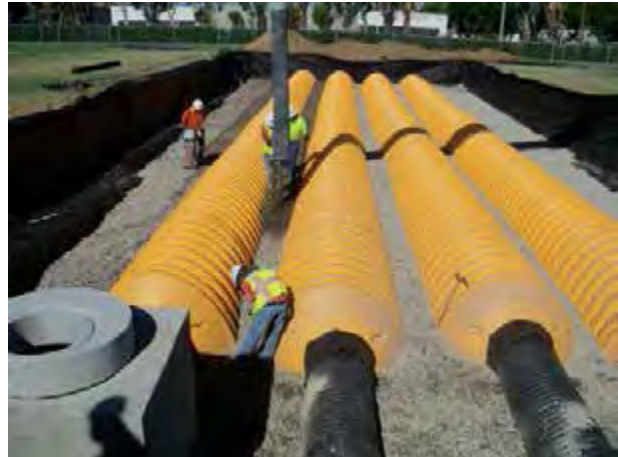
Storm Water Infiltration Structure
