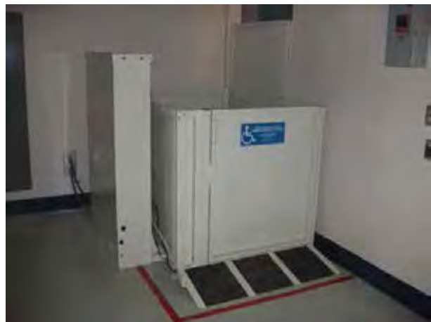
New Wheelchair Lift in the MPR
