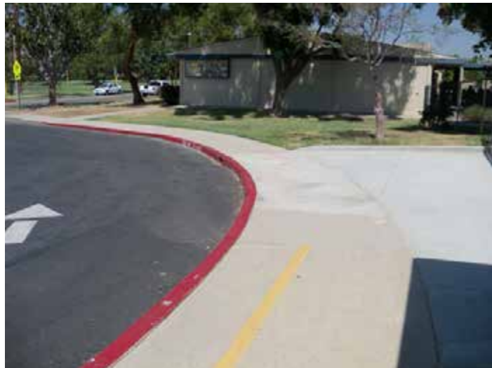
Existing walkway that needs to be corrected (slopes too much side-to-side to meet ADA code)
