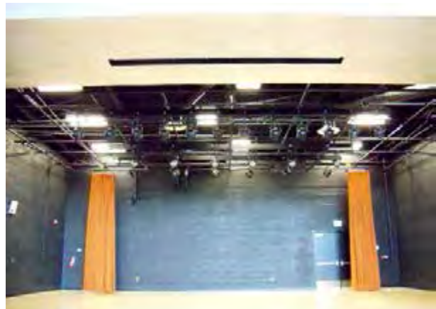
Stage Flood Light Array
