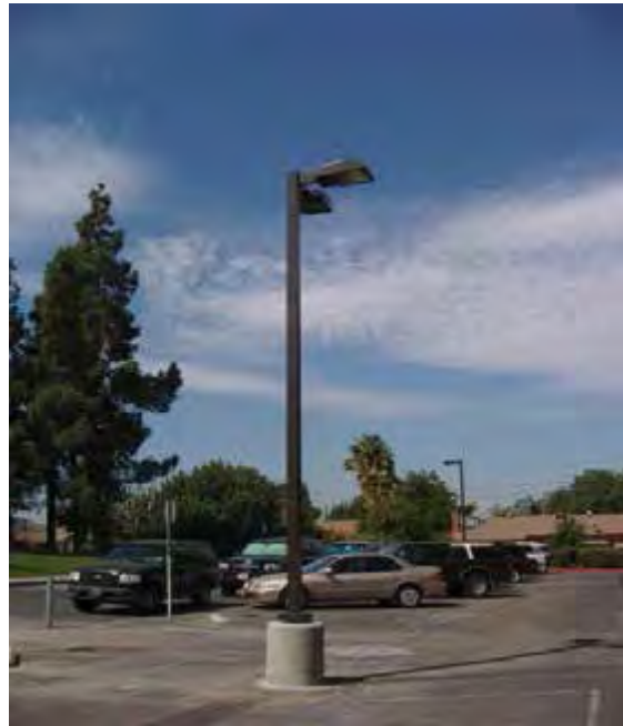
New Parking Lot Lighting
