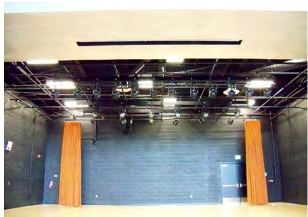
Stage Flood Light Array
