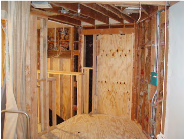
MPR top of stage wheelchair lift platform
