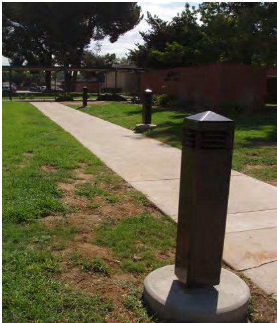
New Illuminated Walkway Bollards
