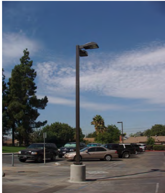
New Parking Lot Lighting
