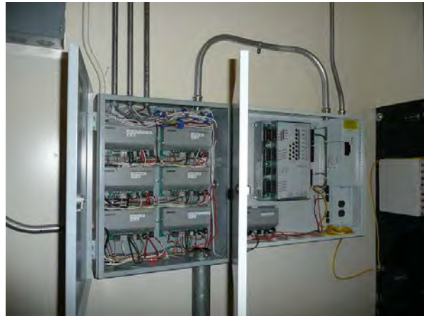
Siemens HVAC and Lighting Controls
