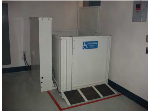
New Wheelchair Lift in the MPR
